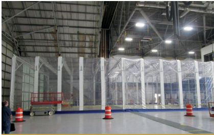
The media blast booth is a steel frame that is wrapped with a clear polyvinyl chloride plastic film.
