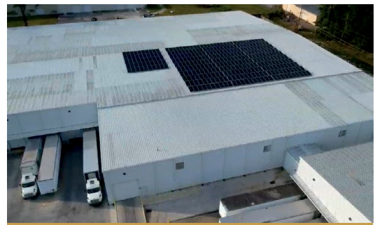
Aerial photograph of the solar panel installation on the roof of Building 3. The rear of the building is located on the upper right side. The area of the incident involved the rear edge of the roof, slightly to the right of the peak. Photo taken and provided by the general contractor.
