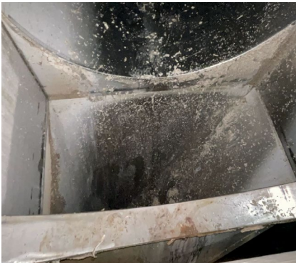
Vertical shaft deceased fell down
